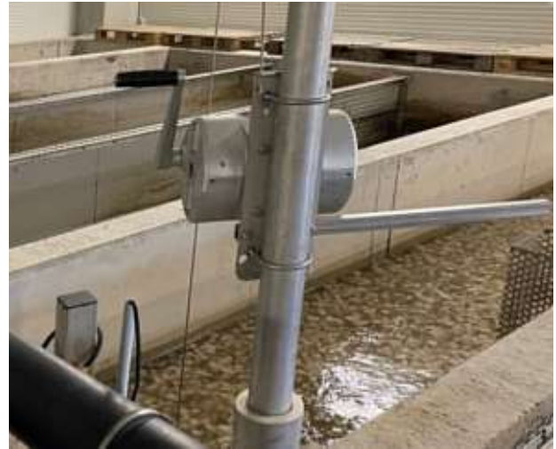
Wastewater treatment by means of Mutag BioChip 30™
